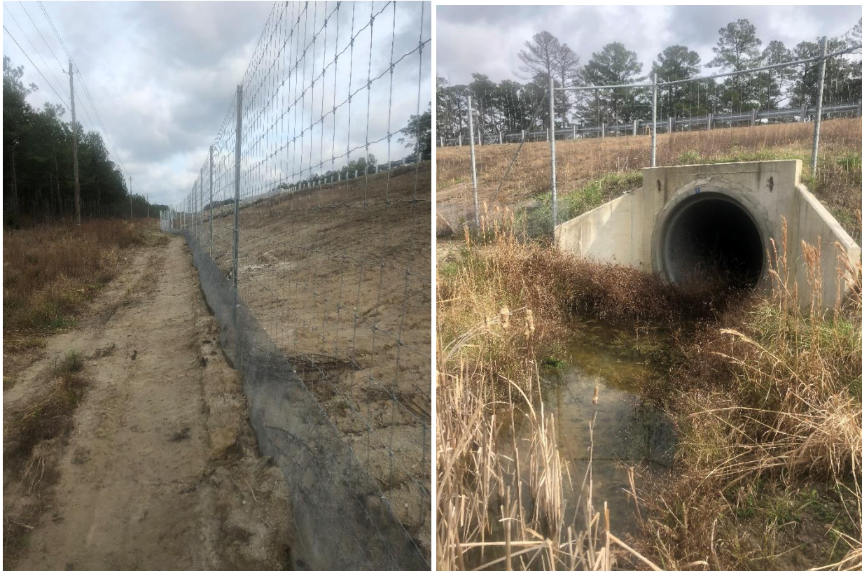
Figures 21 and 22. Wildlife fence run (left) and tie in to crossing structure (right). US 17 Jones County
