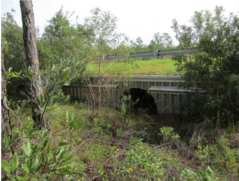
Figure 15. Culvert designed for small and medium animal passage on EF Middleton Blvd. Brunswick County.
