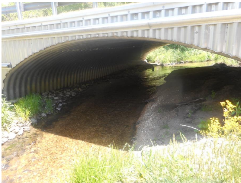
Figure 12. Native material over rip rap backfill in aluminum box culvert (Henderson County, #440073, Greer Creek).
