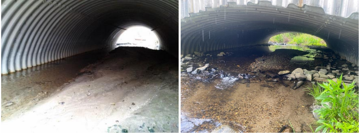
Figures 1 and 2. Wide corrugated metal pipe (Wayne County, SR 1300, Unnamed Tributary) retaining bedload (left) and aluminum box culvert (Transylvania County, , #870163, North Prong Glade Creek) with notched sills and baffles buried by bedload (right, note partially exposed sill in photo right).
